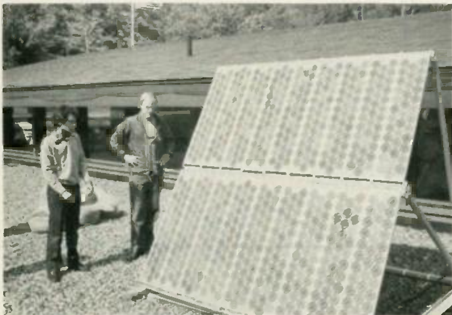
10 PANEL SOLAR ARRAY being installed on the roof of Whiteface Mountain Ski Lodge by Arthur Rudin (left) of Arco Solar, Inc., and Ronald Stewart of the State University of New York, in a project coordinated by the Northeast Solar Energy Center of Cambridge, MA. The solar array will provide power to communications systems for downhill ski events at the 1980 Winter Olympics.
